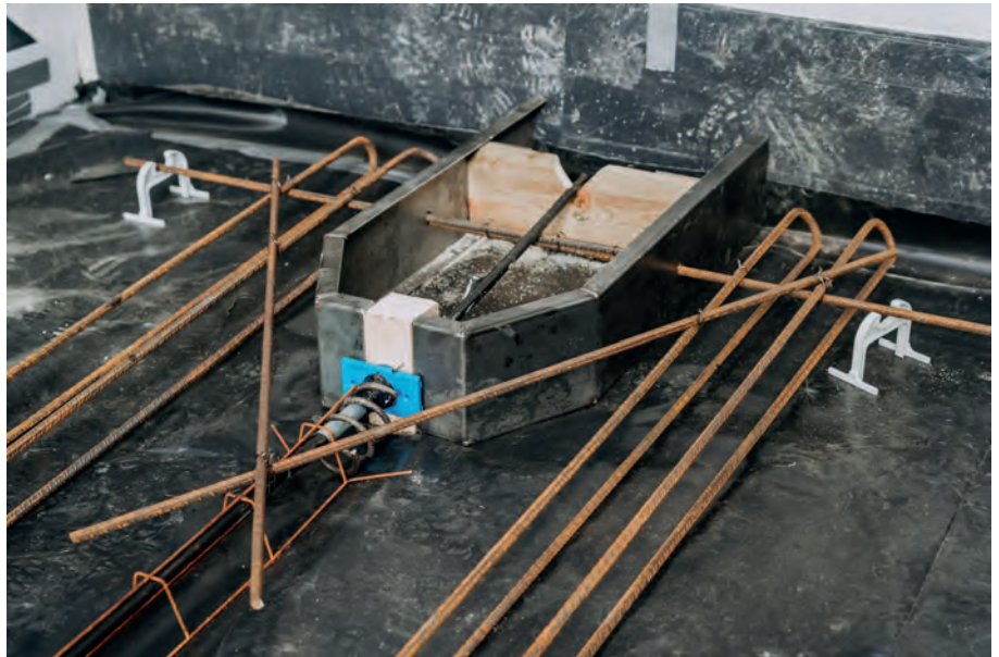
ABOVE: After the stressing pockets were installed, the CCL XU2 anchors were installed and the post-tensioning strands inserted.
